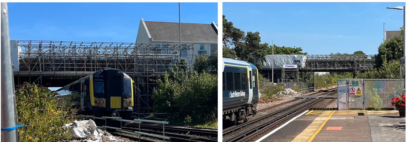
Figure 1: The footbridge with the scaffold structure and tent covering the first section shown from 2 angles.
