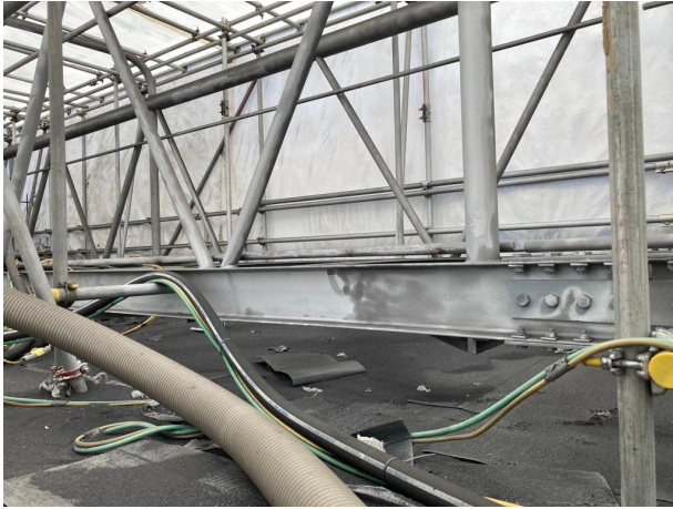
Figure 2: The inside of the tent showing the areas of the bridge that have been shot blasted.
